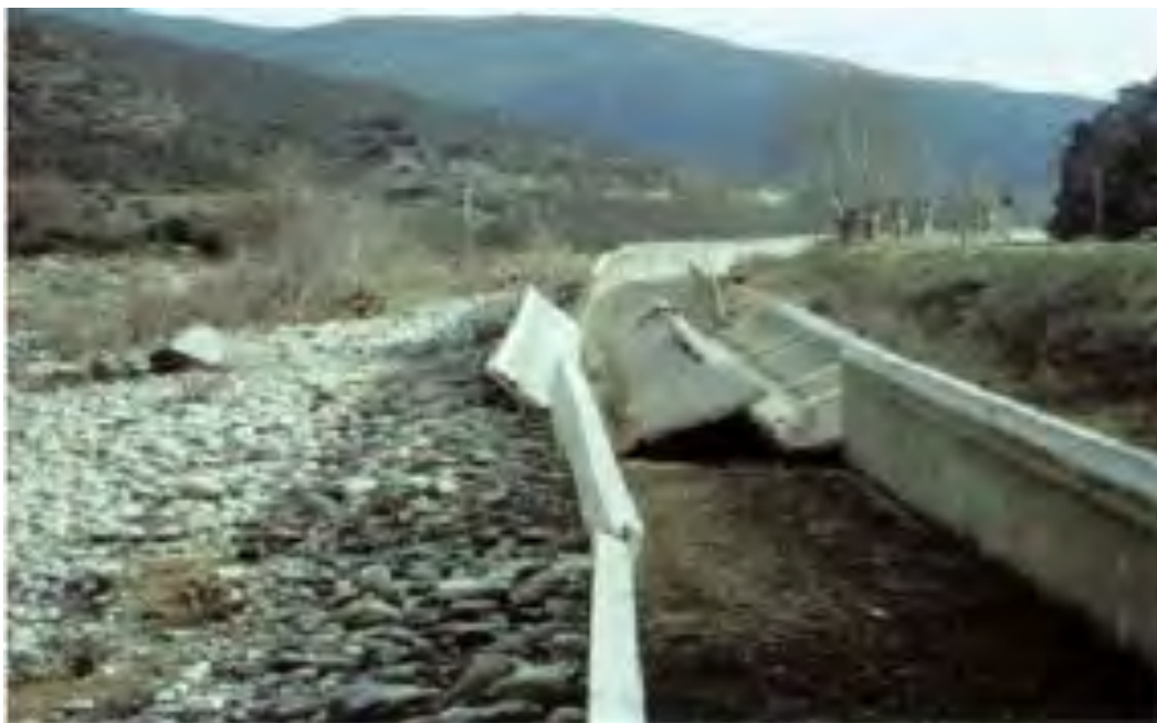
Photo 4-12 Channel destroyed by uplift pressure
