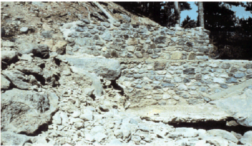
Photo 4-11 Weir undermined by seepage
