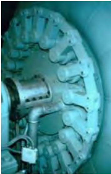
Photo 6.4: Horizontal axis Francis turbine guide vane operating device
