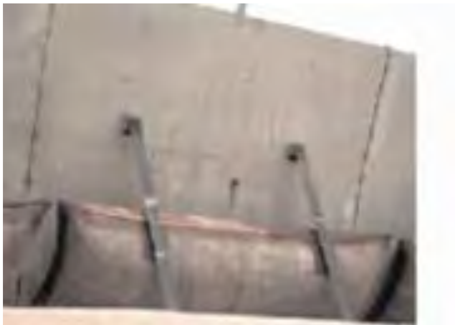
Photo 5.6: Flashboard controlled by inflatable rubber bladder
