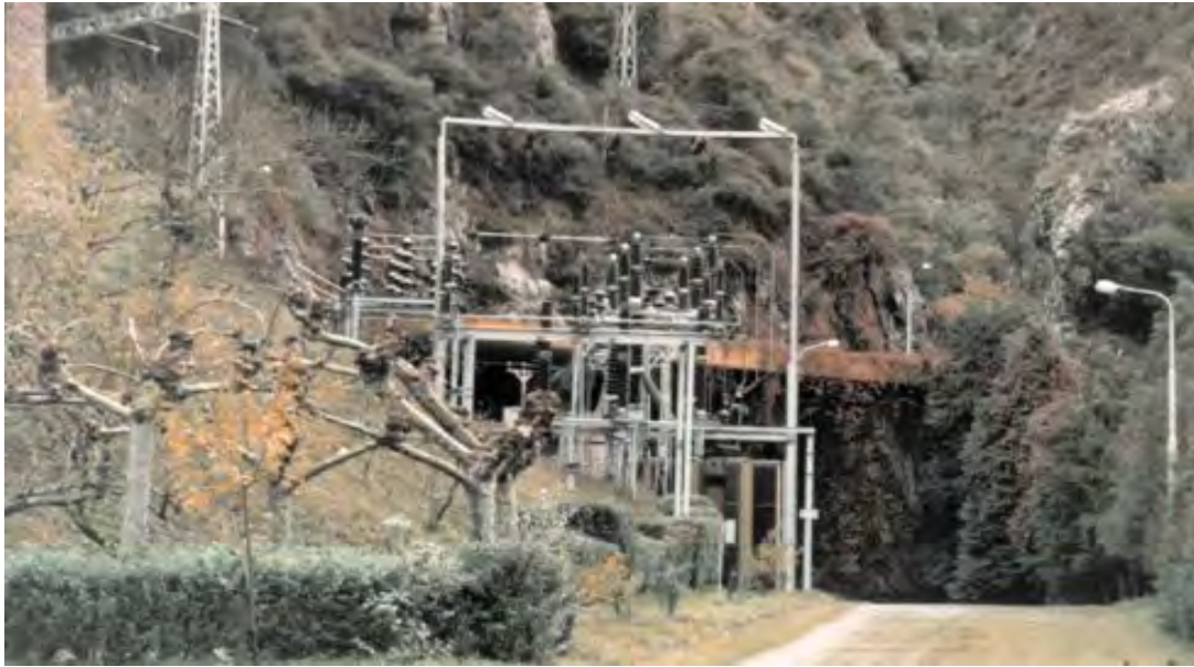
Photo 7.18 Visual impact of outdoors substation
