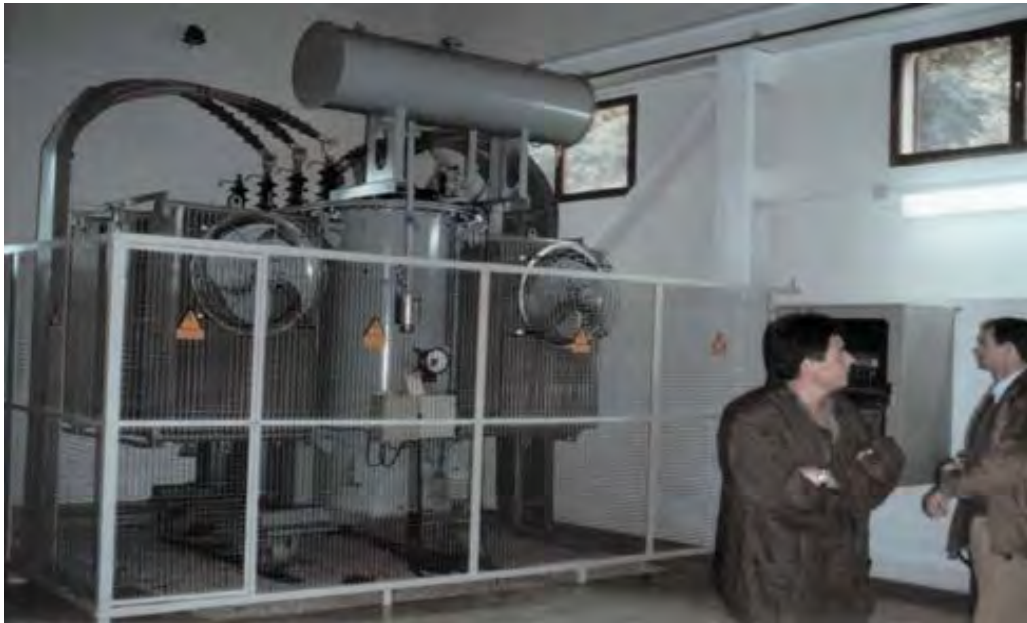
Photo 7.11: Substation located in Powerhouse
